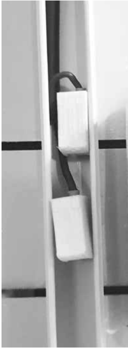
Connection in the cable duct
